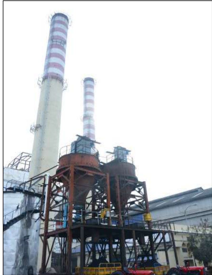
Boiler Ash Handling System
