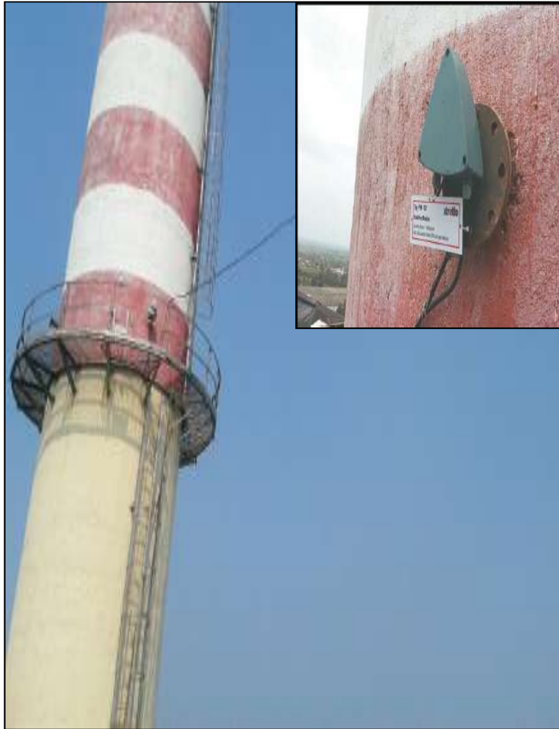
Online Monitoring System
